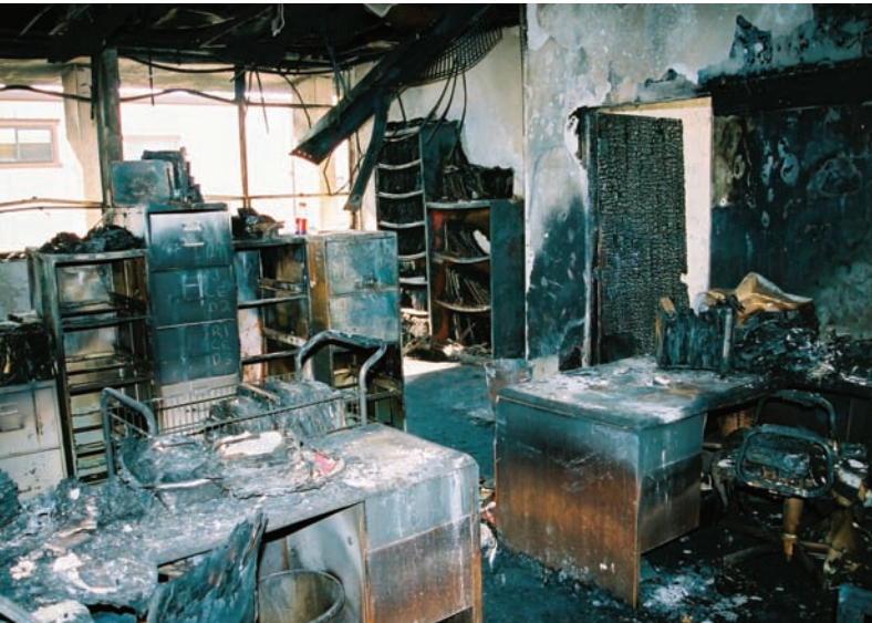
A July 16 fire in the Superior Court of Merced County caused extensive damage to the district attorney's office and blanketed three of seven nearby courtrooms in soot, smoke, and dust.
