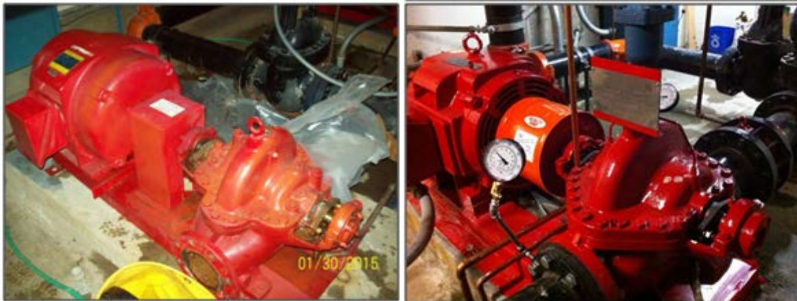
Above (left): One of the old fire pumps. Notice the evidence of leaking seals just above the date stamp on the main pump shaft. Above (right): A new fire pump, installed.
